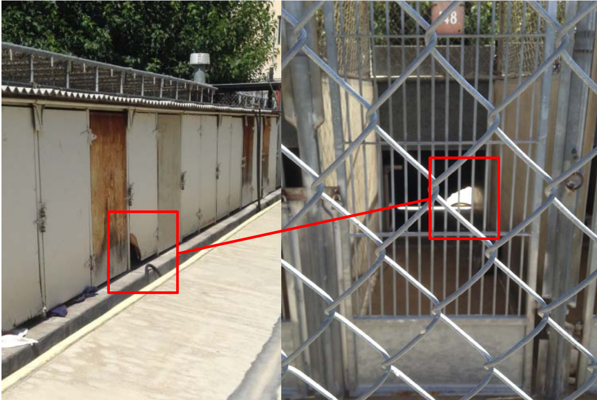
Example of non-functioning kennel due to broken door.
